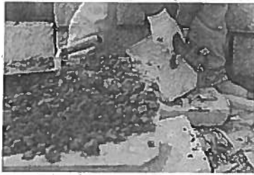
Saul Martinez uses a hammer to even out a cement block while working on a new stone sign at the intersection of Pleasant Hill Road and Satellite Boulevard on Tuesday in Duluth. (Staff Photo: David Welker)
