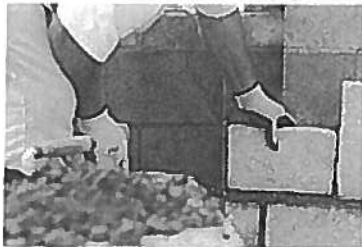
Saul Martinez checks to see if a cement block is flush while working on a new stone sign at the intersection of Pleasant Hill Road and Satellite Boulevard on Tuesday in Duluth. (Staff Photo: David Welker)
